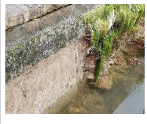
Figure 6. Section of F. enigmaticus removed from canal basin wall
